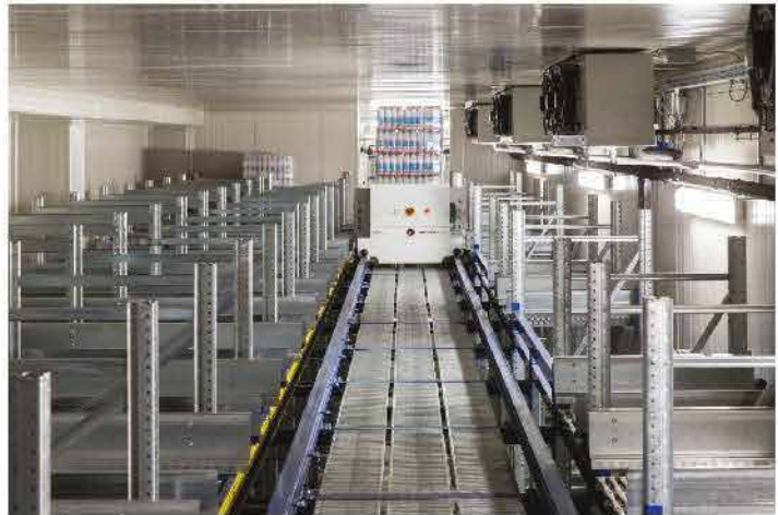
Satellite Storage System Using Automatic Automover
